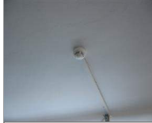
Photo of fire safety equipment Smoke Detector.JPG
