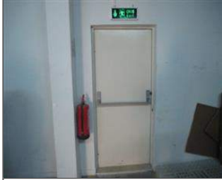
Photo of fire safety equipment Emergency Exit Door (2).JPG
