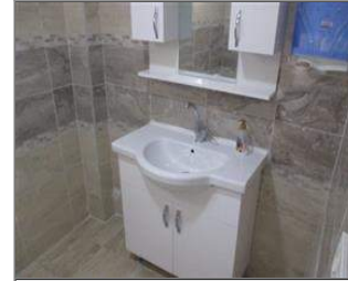
Photo of the sanitary facilities Hand Wash Basin.JPG
