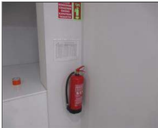
Photo of fire safety equipment Fire Extinguisher.JPG
