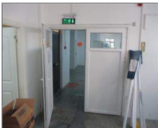
Photo of fire safety equipment Emergency Exit Door (1).JPG
