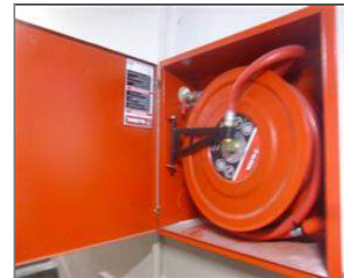
Photo of fire safety equipment Fire Hose.JPG
